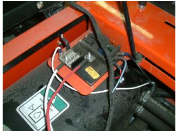
Figure 2: Auxiliary fuse box under seat
